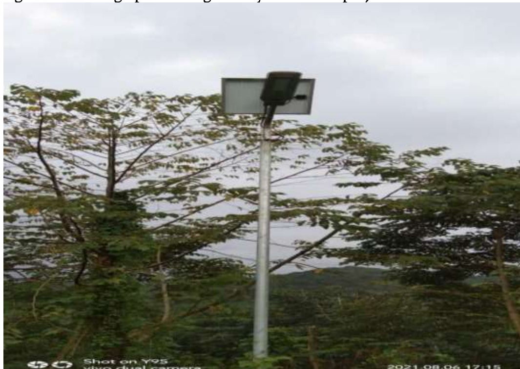
Figure 6 : Photograph showing solar system in the project area
